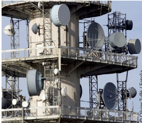
Telecom - Data infrastructure
