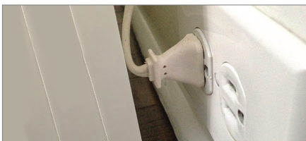
Within electrical cords accidentally damaged by furniture resting or pressing upon them
