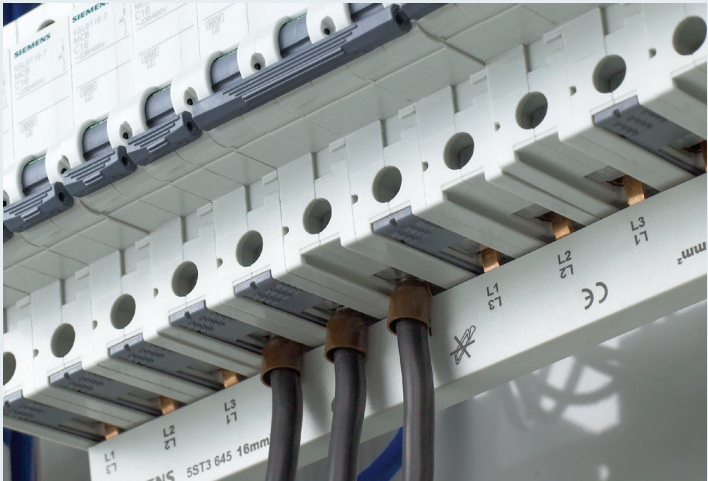
Clearly arranged connection of the supply line in front of the busbar.
